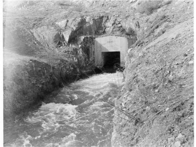
Water flows from the Fire Hill Tunnel above the San Vicente Reservoir San Diego Water Department
