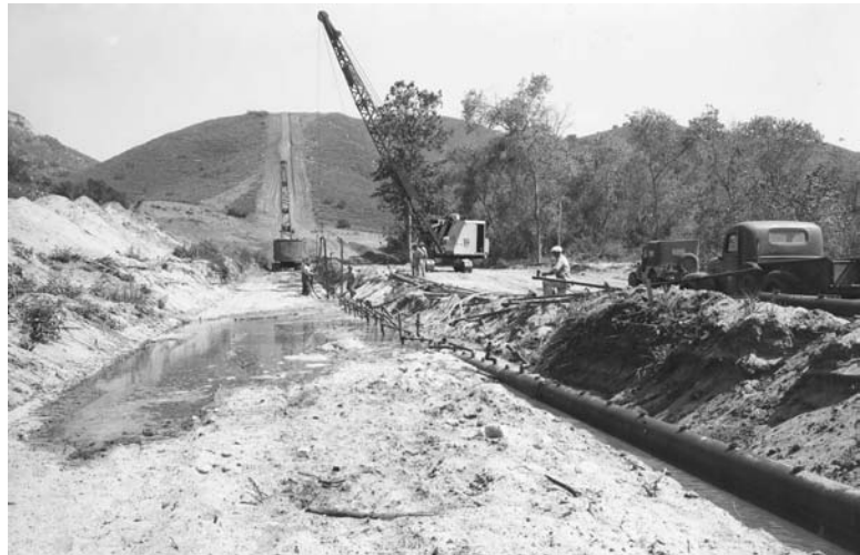
Pipeline construction at the San Luis Rey River, looking south. San Diego Water Department
