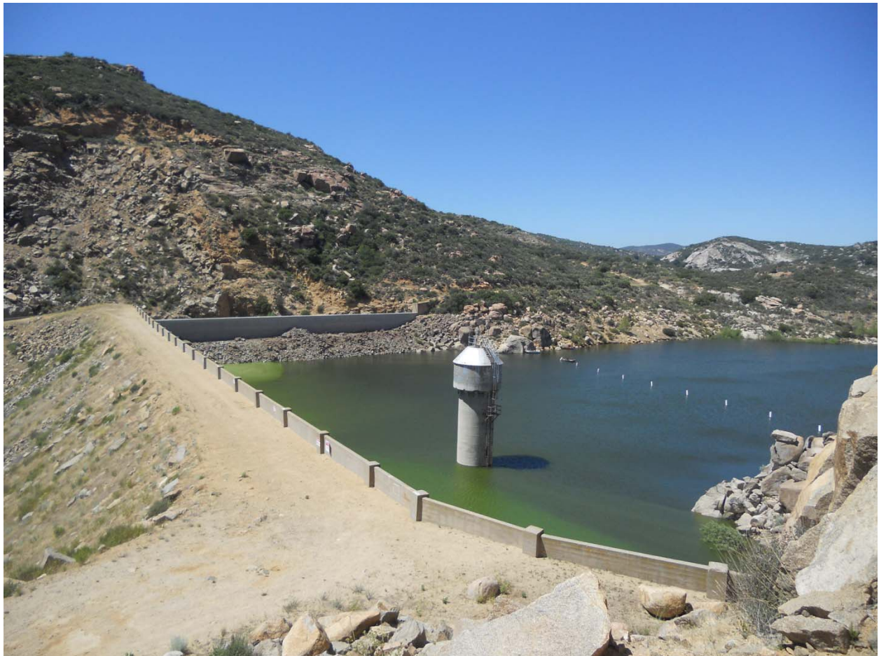
Morena Dam, June 19, 2011. The hills above still show the scars of blasting more than one hundred years ago. The reservoir is at low, 25% capacity. Photo taken by Rick Crawford.
